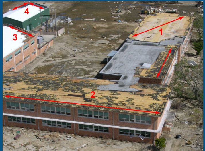
Figure 4. View of damaged school. Four buildings are numbered. Red arrows indicate areas where the roof membrane (Buildings 1-3) or metal roof panels (Building 4) blew off.
